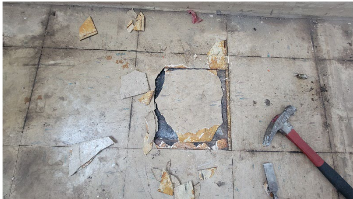
Photo 1 (April 6, 2023): Non-ACM 12"x12" floor tile and mastic (sample sets 008 and 009) over ACM 9"x9" floor tile (sample set 010) and associated mastic (sample set 011) located in the shop restroom.
