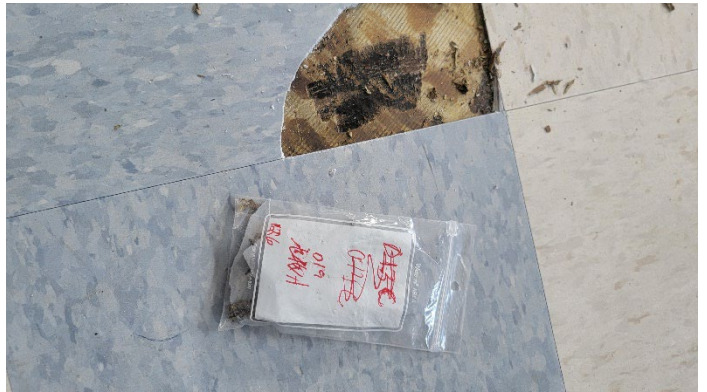
Photo 2 (April 7, 2023): ACM tan/black mastic (sample set 016ABC) beneath non-ACM 12"x12" floor tiles on the first and second floors of the 1968 addition.
