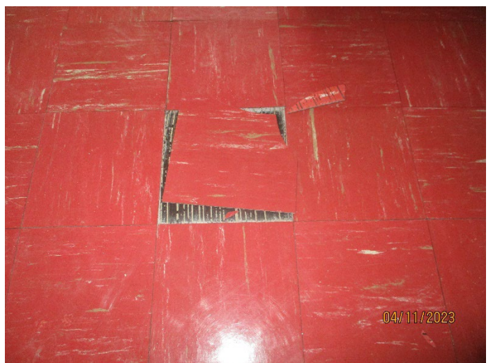
Photo 6 (April 11, 2023): ACM 9"x9" red floor tiles (sample set 053) located on the first floor of the 1968 addition.
