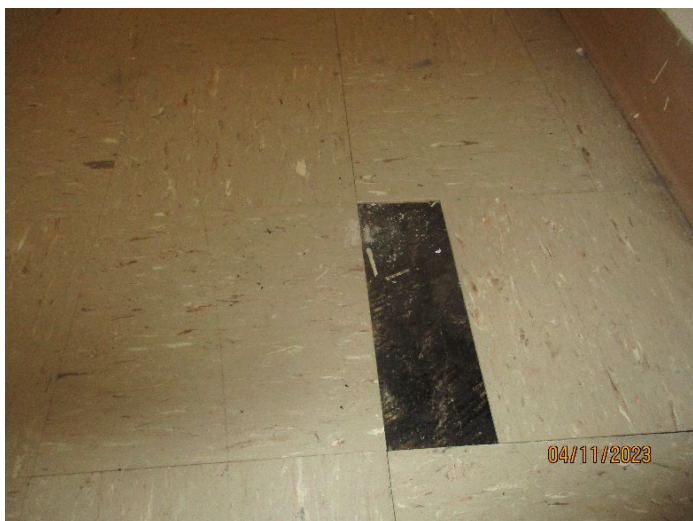
Photo 5 (April 11, 2023): ACM 9"x9" floor tiles (sample set 052) located on the second floor of the 1968 addition.
