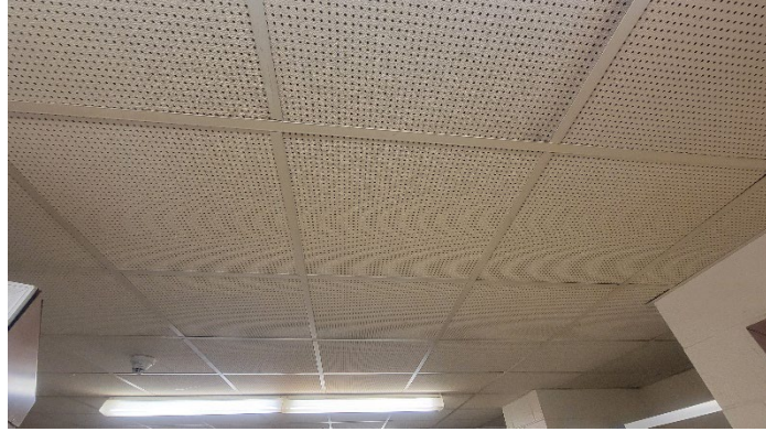
Photo 1 (April 6, 2023): PACM ceiling tiles located in the girl's locker room of the 1968 addition.
