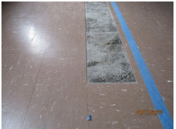
Photo 4 (April 11, 2023): ACM residual mastic (sample set 032) and ACM 9"x9" brown floor tiles (sample set 051) located in the first and second floor hallways of the 1968 addition.
