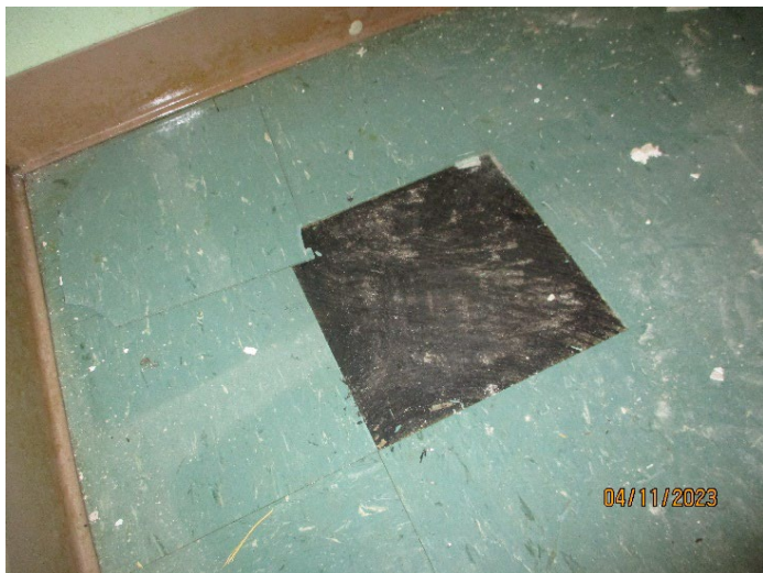
Photo 3 (April 11, 2023): ACM 9"x9" floor tile (sample set 049) and associated mastic (sample set 050) located in the second-floor band room closets in the 1968 addition.
