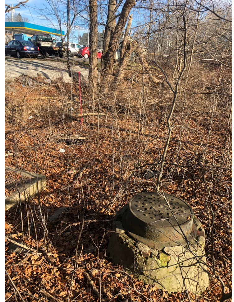
Cross Country Sewer
